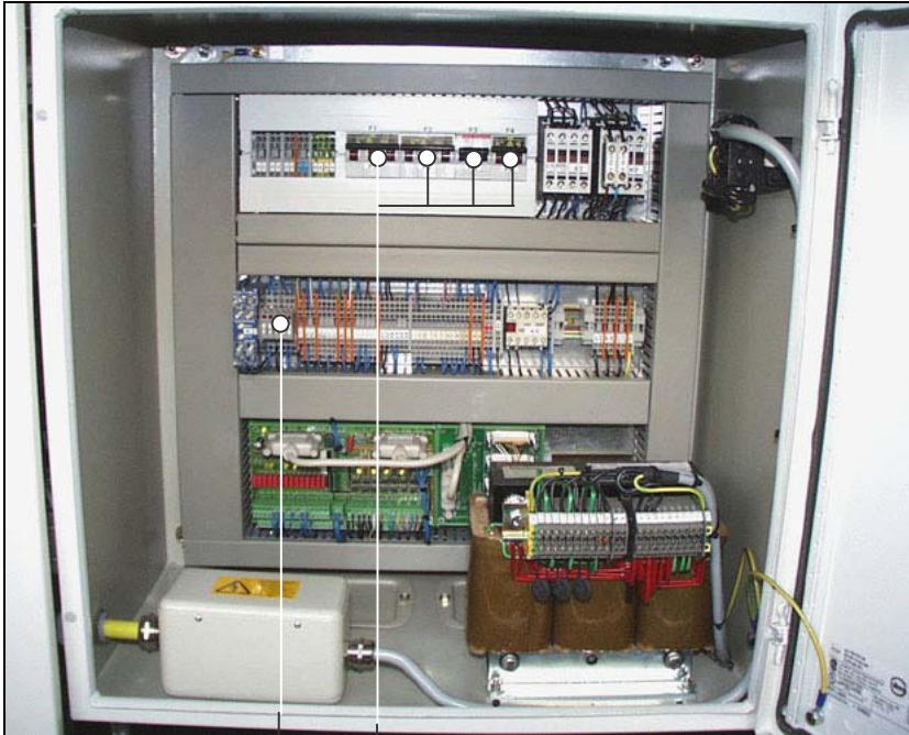
Fuses Switch Cabinet
